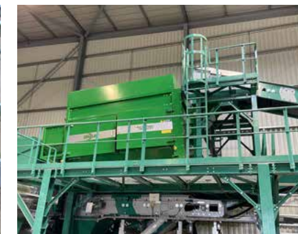
MS 5200-ST Integrated into a processing line
